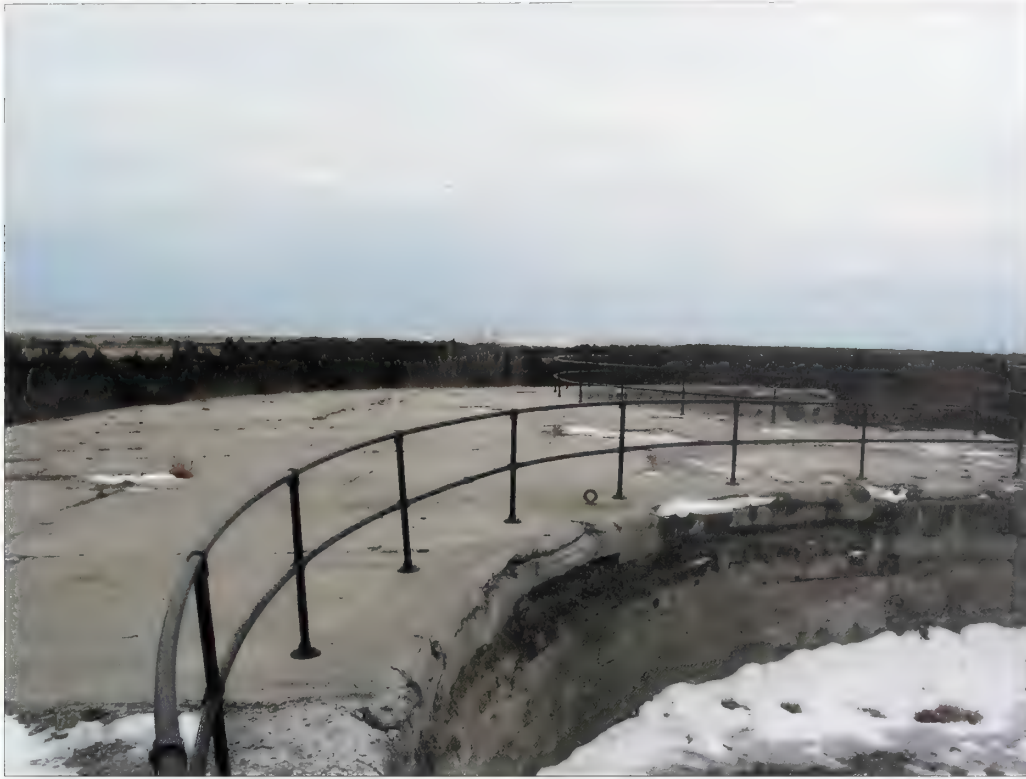
Figure 3.29. View looking south at guardrails, Battery Potter. To increase visitor safety, the National Park Service has recently added guardrails between the superior slope and the terreplein where the guns were emplaced (Olmsted Center, January 2009).
